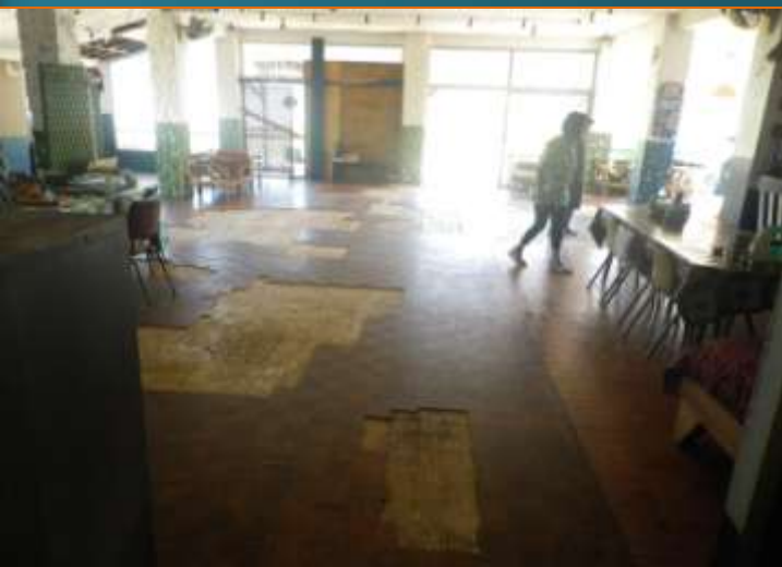
Below: After Cyclone PAM and after repairs
