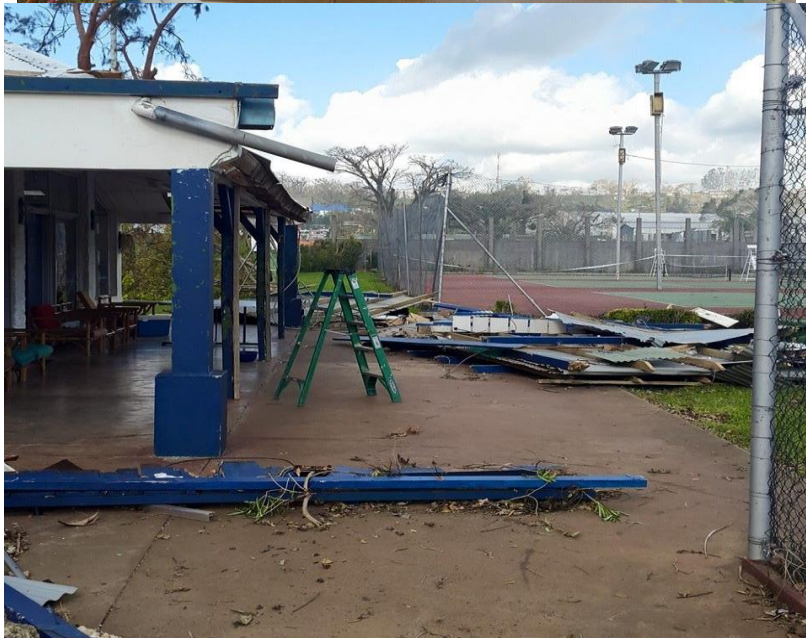
14.03.2015. Club House: external terrace is gone
