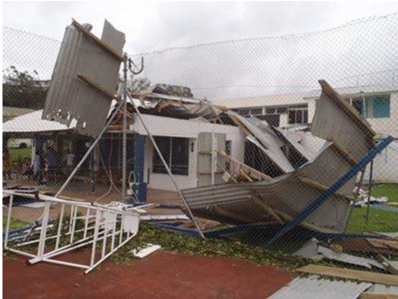
15.03.2015. Part of the roof blown on to court 3
